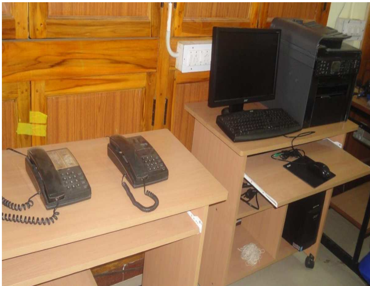
The Land line and Toll Free 1077 telephone connections in DEOC
