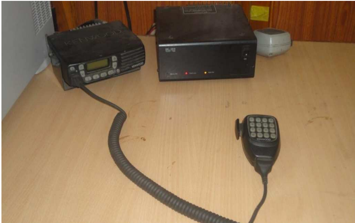
Communication Equipments in DEOC, Viluppuram
